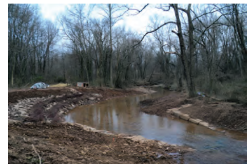
Newly constructed sloping streambanks will be planted with dogwood and willow trees to resist erosion.
