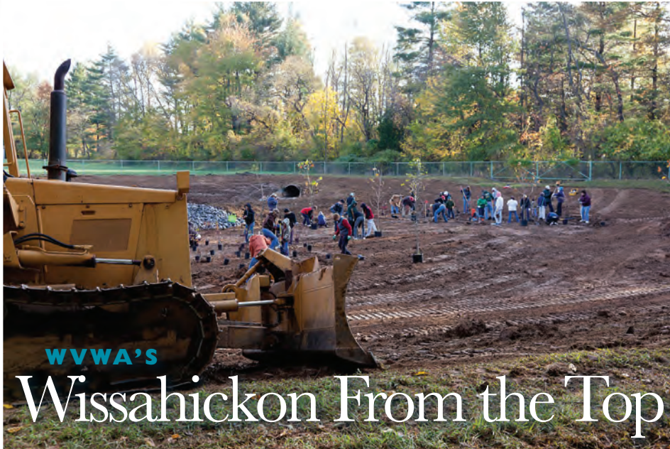
Utilizing volunteer labor and heavy equipment, a 2010 project retrofitted a storm water basin on North Wales Road in Upper Gwynedd.
